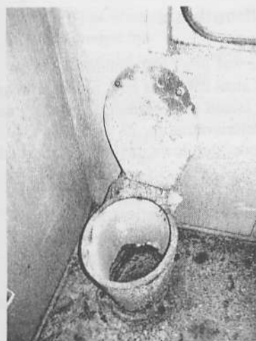
The original toilet, which would simply dump human waste onto the tracks, is intact.
